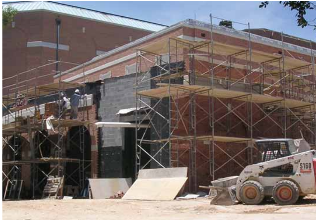
Workmen strive to complete the exterior of Samford's new recital hall, set to open this fall.
