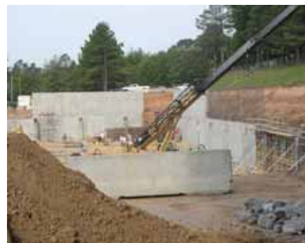
Builders work on foundational walls for Pete Hanna Arena May 26. Go to www.samford.edu for progress updates.
